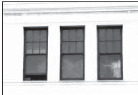
Double hung windows were common on the upper floors of commercial buildings.
