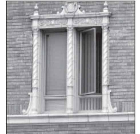
Metal casement windows were also common on upper stories in commercial buildings.
