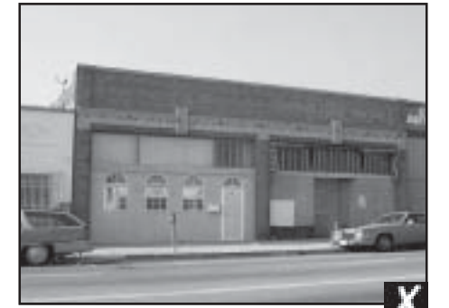
Filling in storefront windows dramatically changes the character of a commercial building
