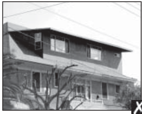
This rooftop addition is inappropriately located on the side of the house.
