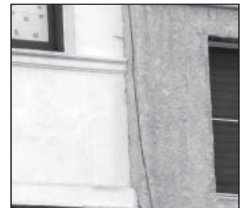
The smooth stucco finish on the left approximates the original historic finish, while the rough finish on the right is not historic.
