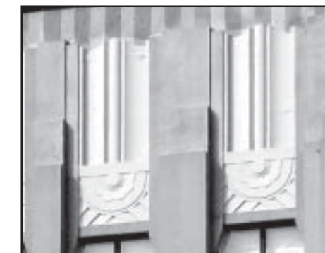
Concrete detail like this should not be cleaned with aggressive abrasive methods, or the detail may be lost.
