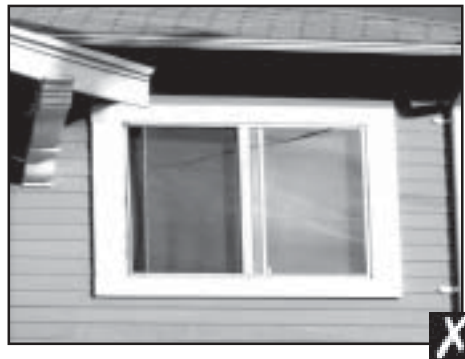
These sliding aluminum replacement windows are inappropriate.
