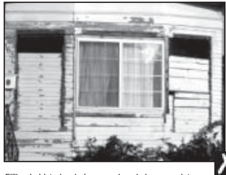
Filling in historic window openings is inappropriate.
