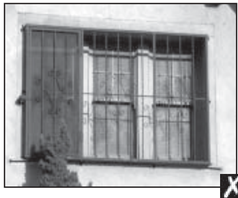
These security bars obscure the historic windows behind
