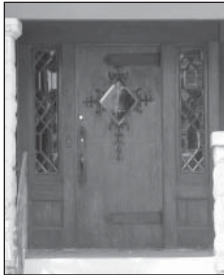
Loss of this door and its sidelights would have a negative effect on the character of this house.
